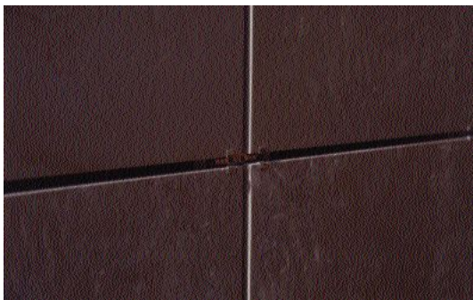
Sistema FV anclaje visto. FV system with visible anchoring.
